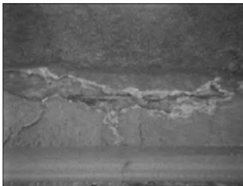
Major Damage to Fire Insulation
