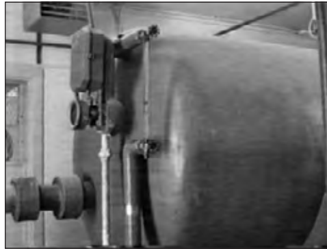
Boiler or vessel insulation
